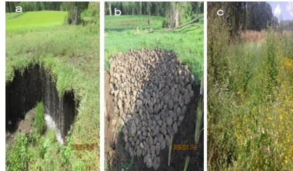
Fig. 1. Gully head protection: a) before gully control structure in place; b) immediately after regrading and placement of stone riprap (June 2015); and c) after 4 months of the rainy season (October 2015) well stabilized and covered with vegetation.
