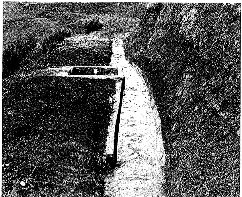
Figure 8.1.4. Ten-meter section of lined canal at the intake and the pipe inlet box.
