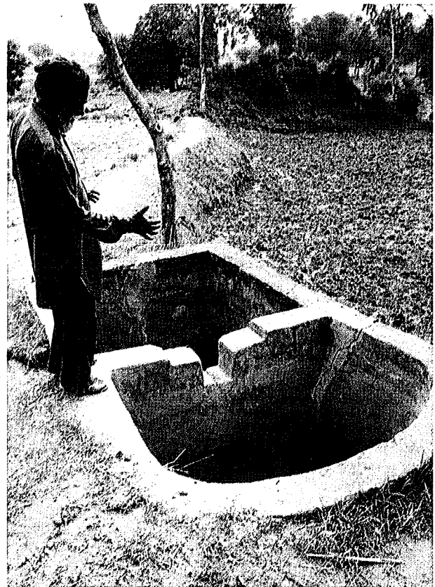
Figure 7.8.1. Discharge regulator for pressurized distribution system in Haryana, India.
