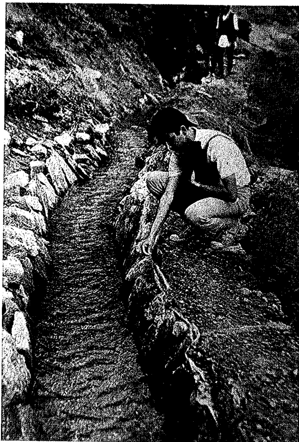
Figure 6.0.7. Plastic sheet used to reduce seepage from a canal in a landslide zone in Sindhupalchok, Nepal.
