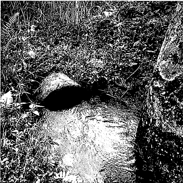
Figure 4.2. Partially blocked pipe.
